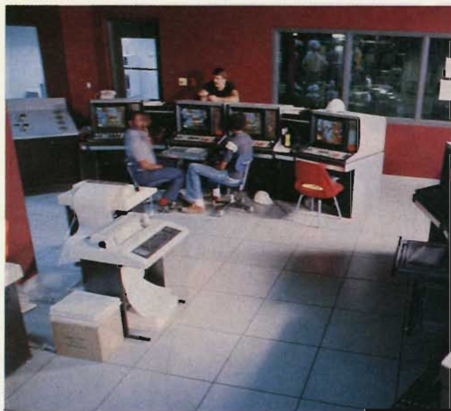
Figure 6 — Control room for a large distributed-control system
